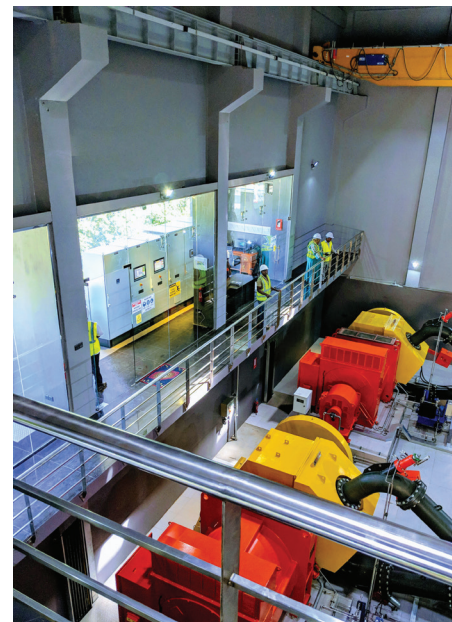
Above: Turbine Generators & Control Room at Lubilia
